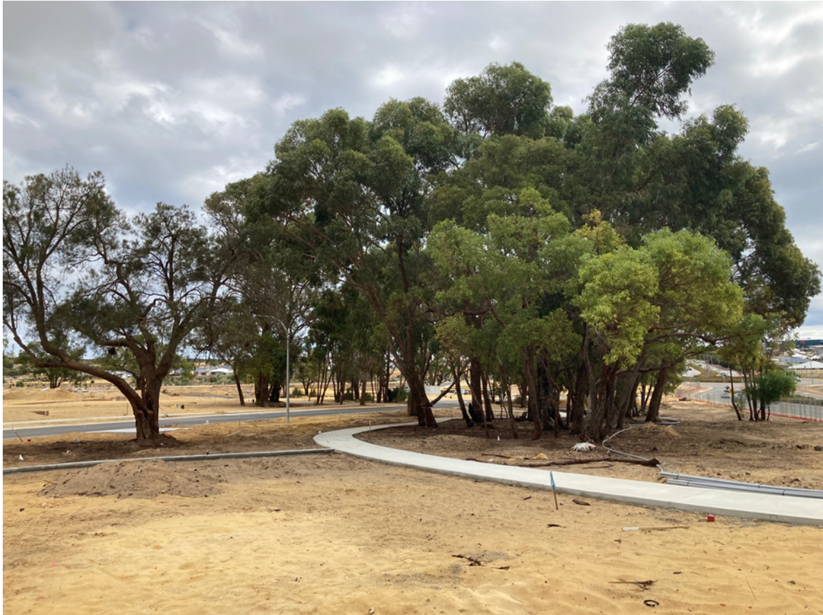
Catalina Green Public Open Space corner Neerabup Road and Connolly Drive - Construction commenced
