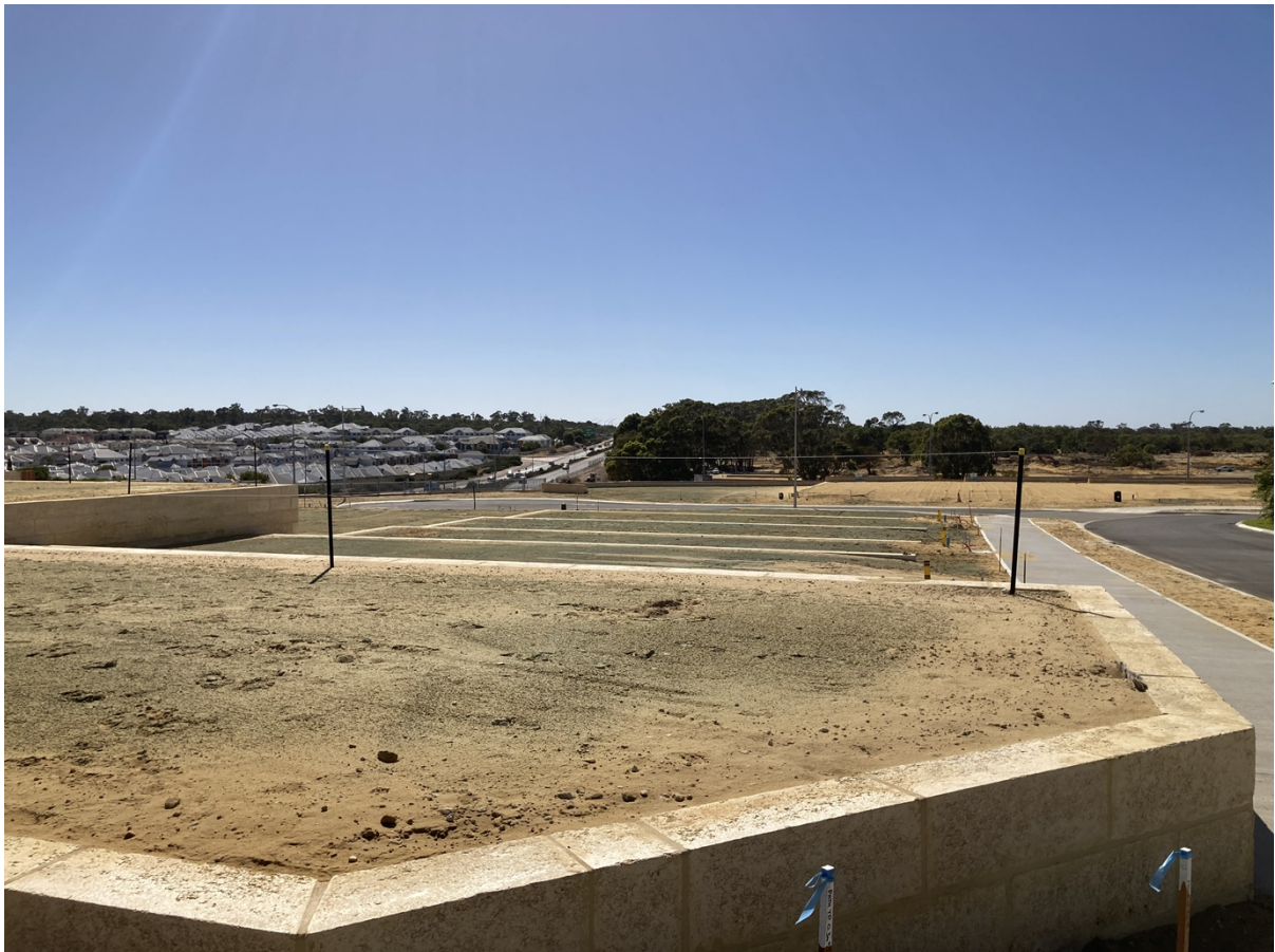
Completed Stage 18C lots in Catalina Central, looking east towards Stage 36 in Catalina Green
